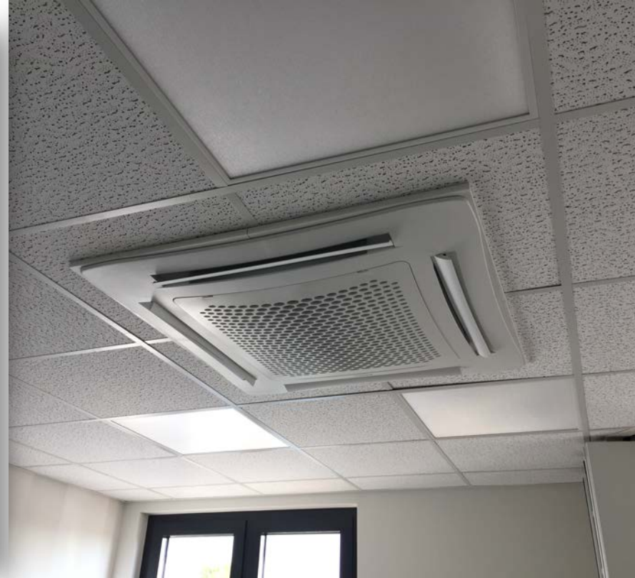
Fan Coil Control-Room
