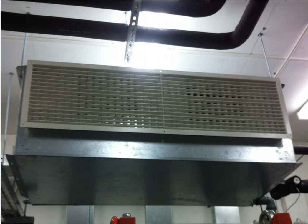
Fan Coil UPS-Room
